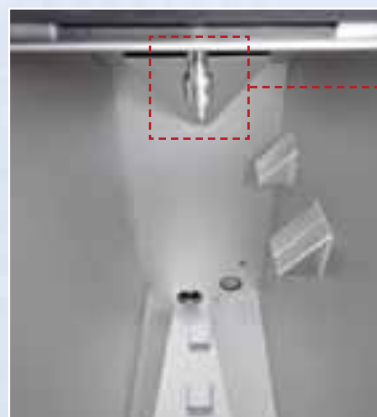
Rotating cleaning nozzle in cockpit recovery tank
